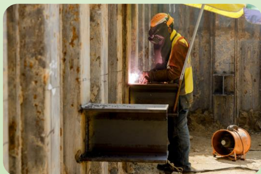
新建污水處理廠的挖掘及側向支撐安裝工程 Excavation and Lateral Support (ELS) Works for the New Sewage Treatment Works
