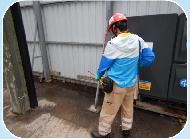
在工地周邊進行消毒以預防2019冠狀病毒病 Sanitizing the Surroundings of Site to Combat COVID-19 Pandemic
