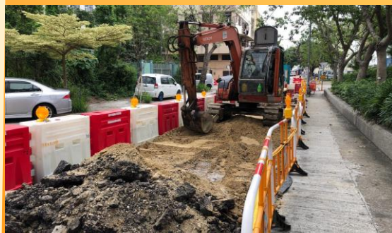
塘肚村及沙頭角墟污水渠鋪設工程 Construction of Sewers at Tong To Village and Sha Tau Kok Town
